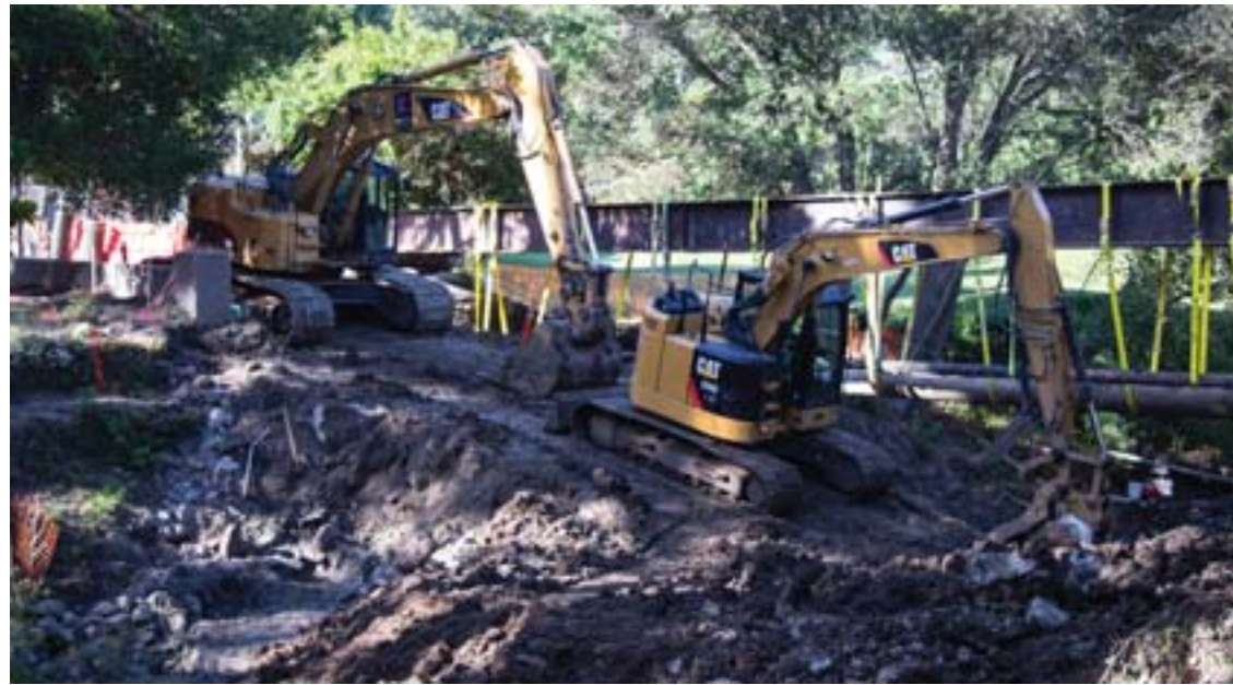
Orinda is bringing in equipment to start the repairs to the Miner Road sinkhole.
